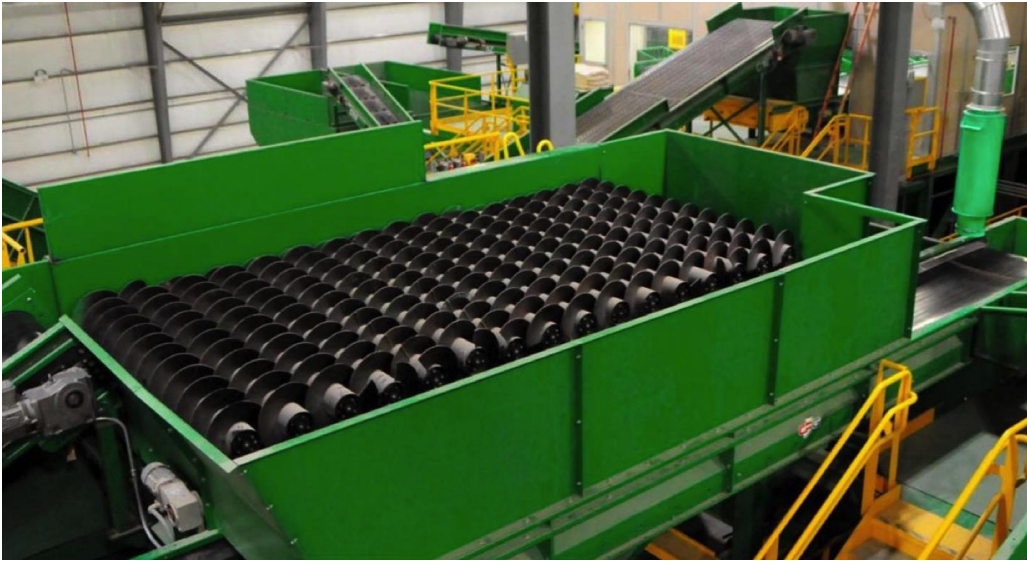
Figure 23 CP Auger Screen (B)
