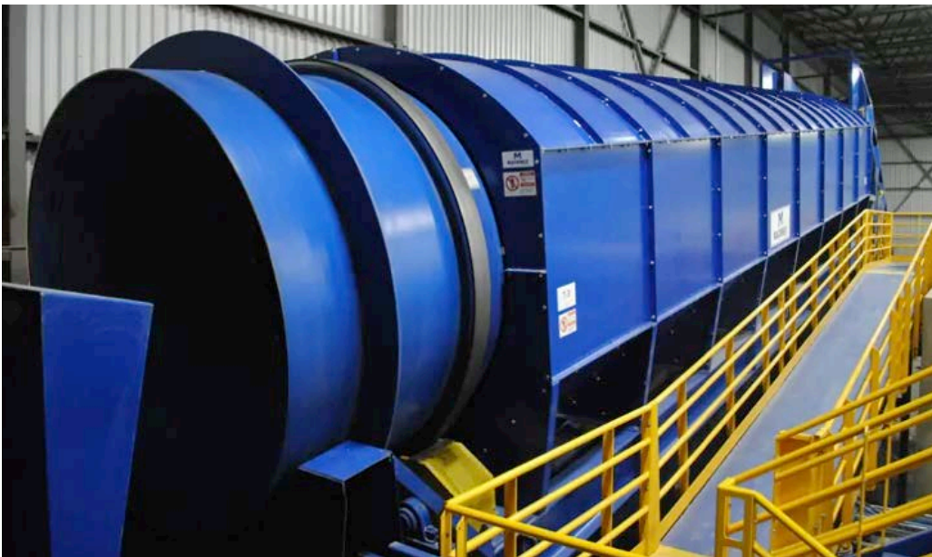
Figure 24 Machinex Trommel (C)
